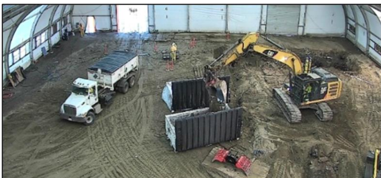
Click here for a time lapse video of remediation activities inside the structure.
